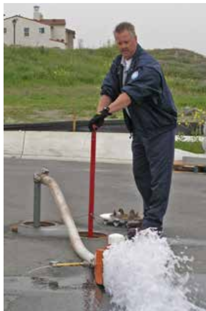
A water main valve is opened by Water Systems Operator Jim Killips to flush out natural sediments that build up over time.
