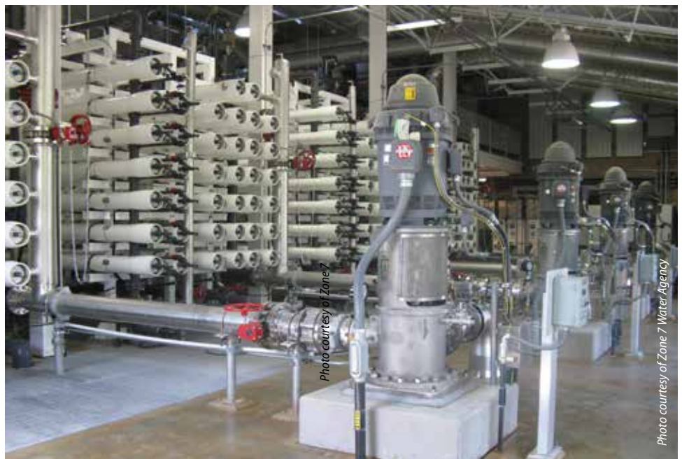
Zone 7's Mocho Well Demineralization Plant in Pleasanton.
