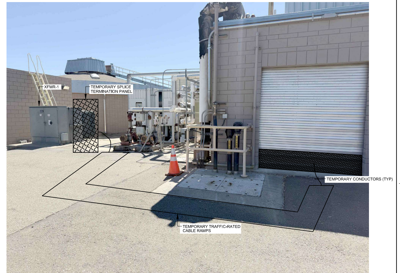
EXTERIOR FROM GENERATOR ROOM ROLL-UP DOOR TO TEMPORARY TERMINATION SPLICE PANEL
