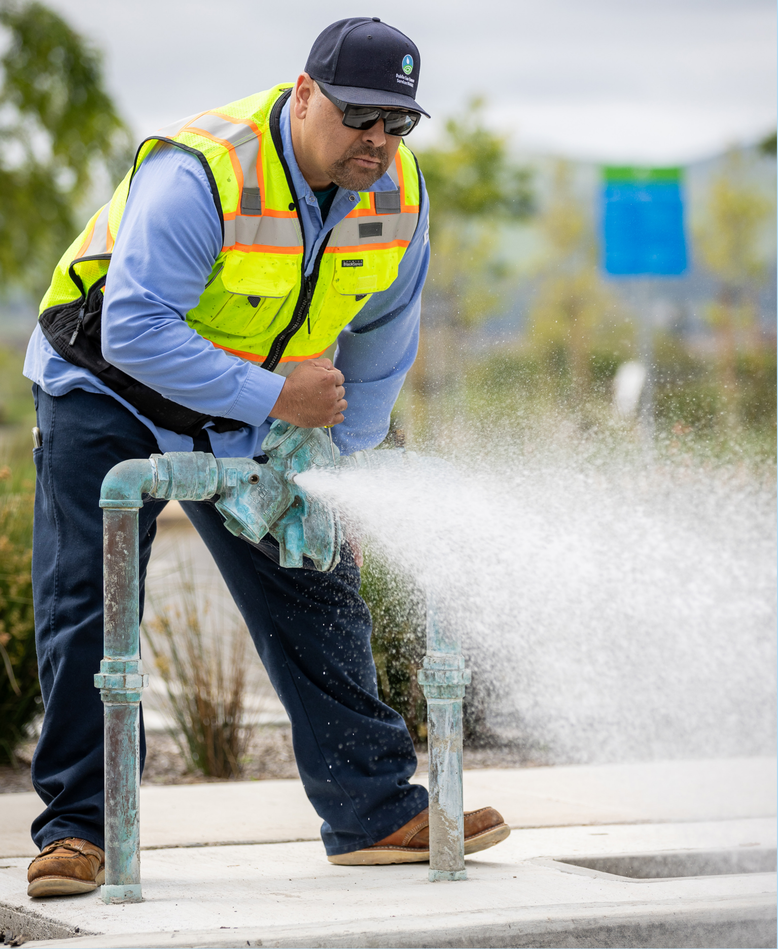
A DSRSD employee opens a test cock on a backflow prevention device to verify that it is receiving water flow.
