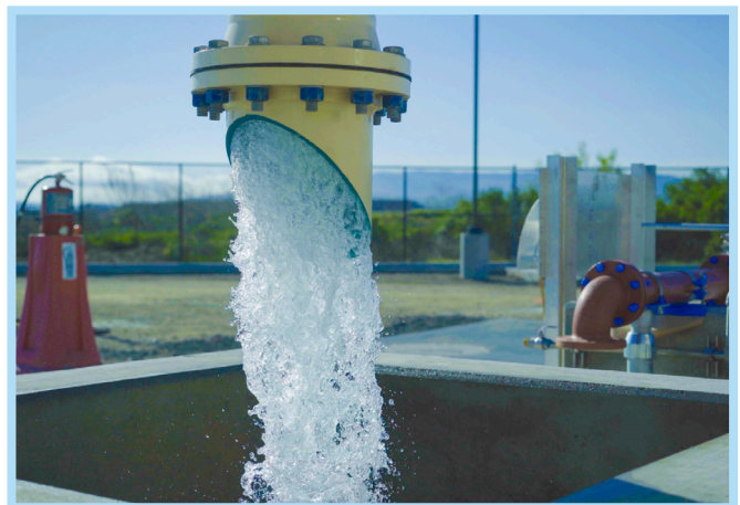
Zone 7 operates multiple wells that extract groundwater to supplement your water supply. Photo courtesy of Zone 7 Water Agency.
