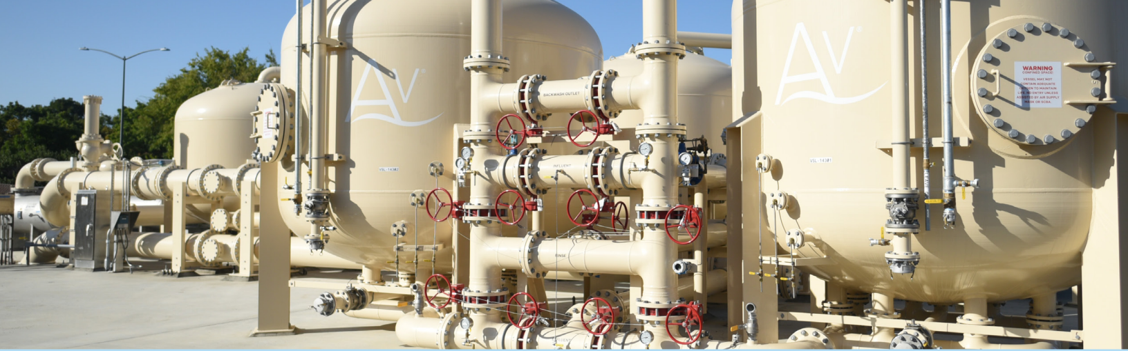
Zone 7 uses ion exchange to remove PFAS for our water supply. Photo courtesy of Zone 7 Water Agency.
